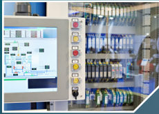
IPC & HMI Panels
